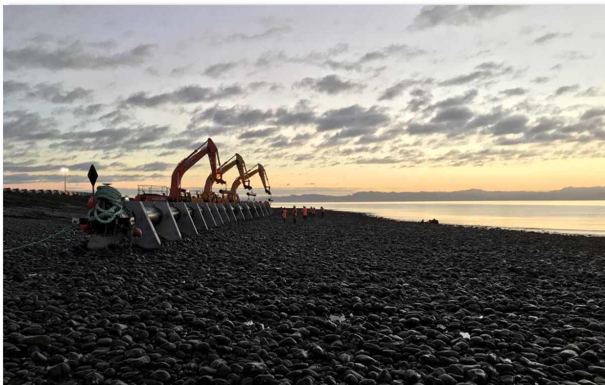
The 450m long seabed pipe string at Kaiaua, before it was towed to Army Bay
