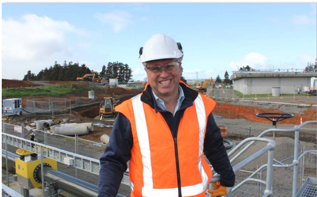
Project manager, Sven Harlos at the Pukekohe wastewater treatment plant upgrade construction site
