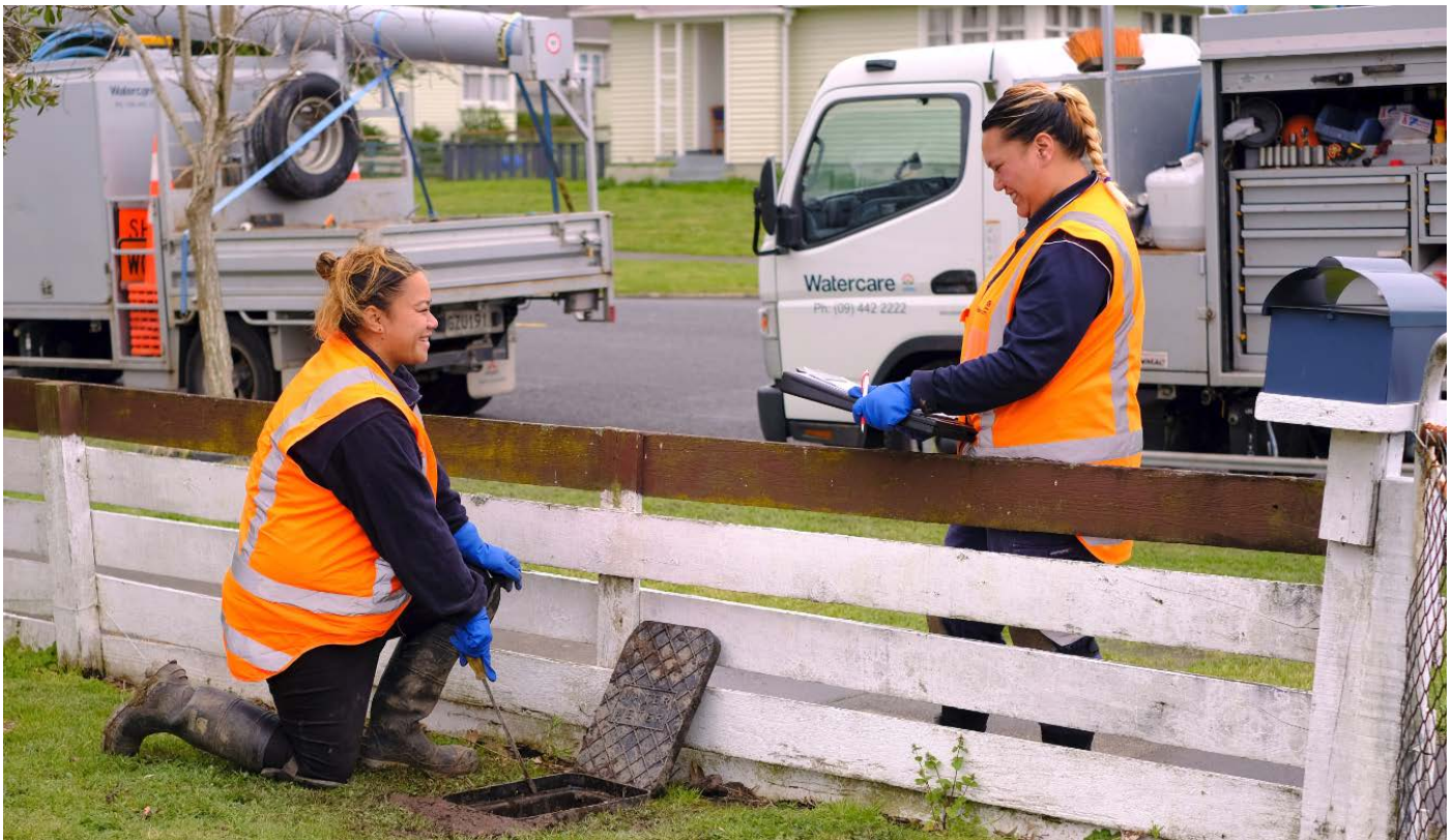
Watercare Maintenance Service Network servicepeople, Rangz Elliot and Rangz Fenton, working on the planned meter replacement programme
